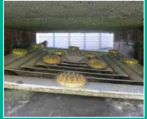
Air Conditioning Vents
