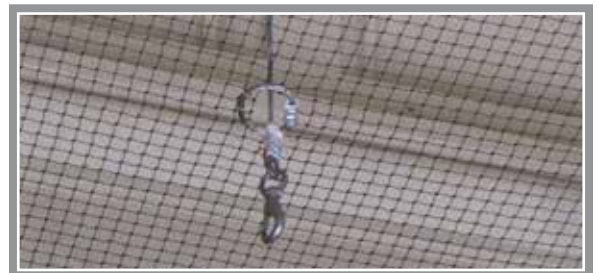
StealthNet installed horizontally under a courthouse ceiling. The cable and clip allows workers to attach banners below the netting.
